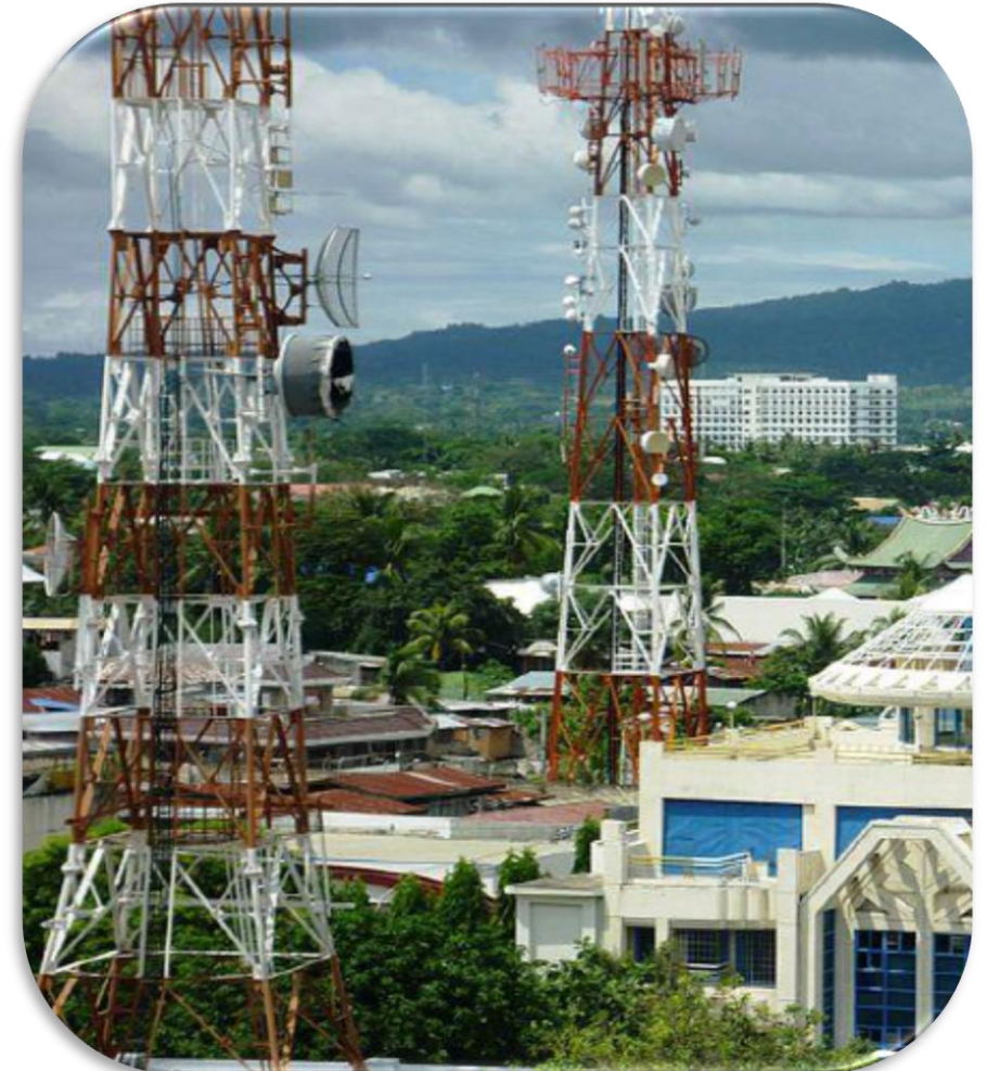
Telecom Towers (Representational)
